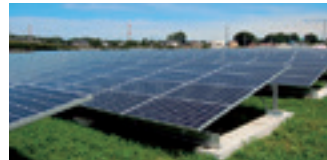
Tsurugashima Photovoltaic Power Plant (Tsurugashima-shi, Saitama Prefecture)
