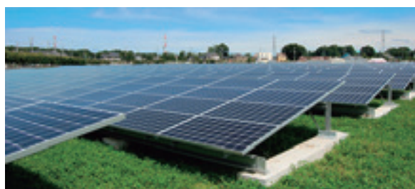
Tsurugashima Photovoltaic Power Plant
